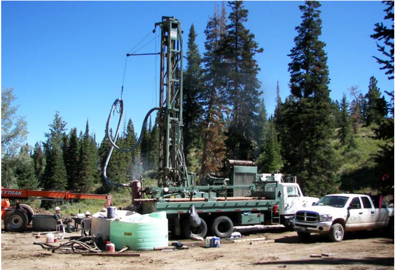
Drilling 1,500 foot Water Test Well on the East side of Sharp Mountain
